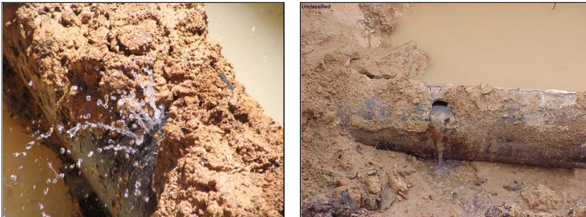
Figure D-16. Fire Protection Lead-In Piping Corrosion.
